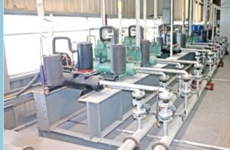
Refrigeration test system
